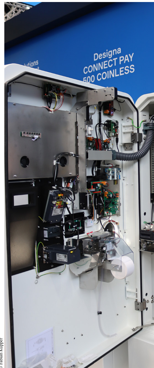
The inner workings of a parking ticket machine.
